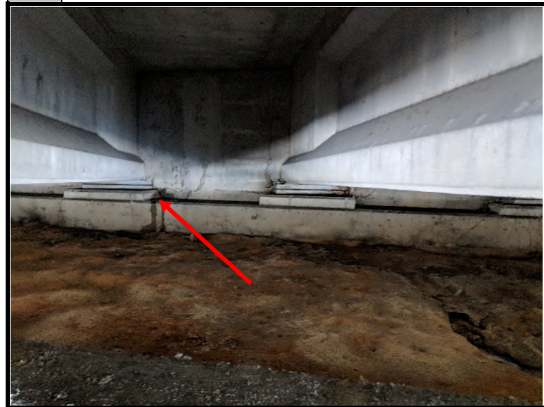
4 The felt paper beneath bent plates tested negative for asbestos via PLM and TEM analysis. The gray bent plate tested positive for lead-based paint (23.00 mg/cm 2 ).
