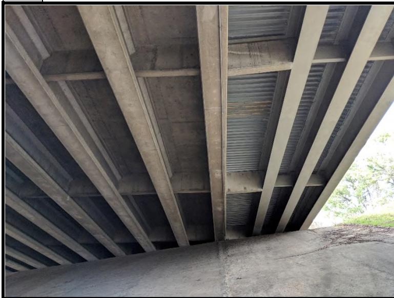
3 View of the underside of the bridge. Shows concrete beams and metal decking on center lanes and steel beams with metal decking on outside lanes.
