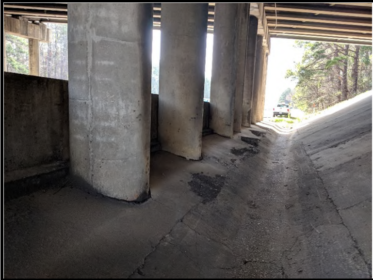
5 Expansion joint located around base of columns tested negative for asbestos via PLM and TEM analysis.
